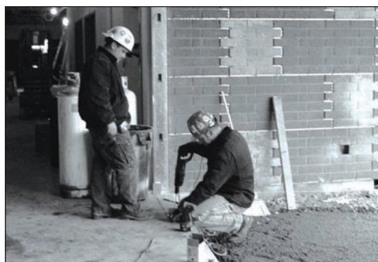
James Tennis (left) and Ryan Penning work on the new science building.
