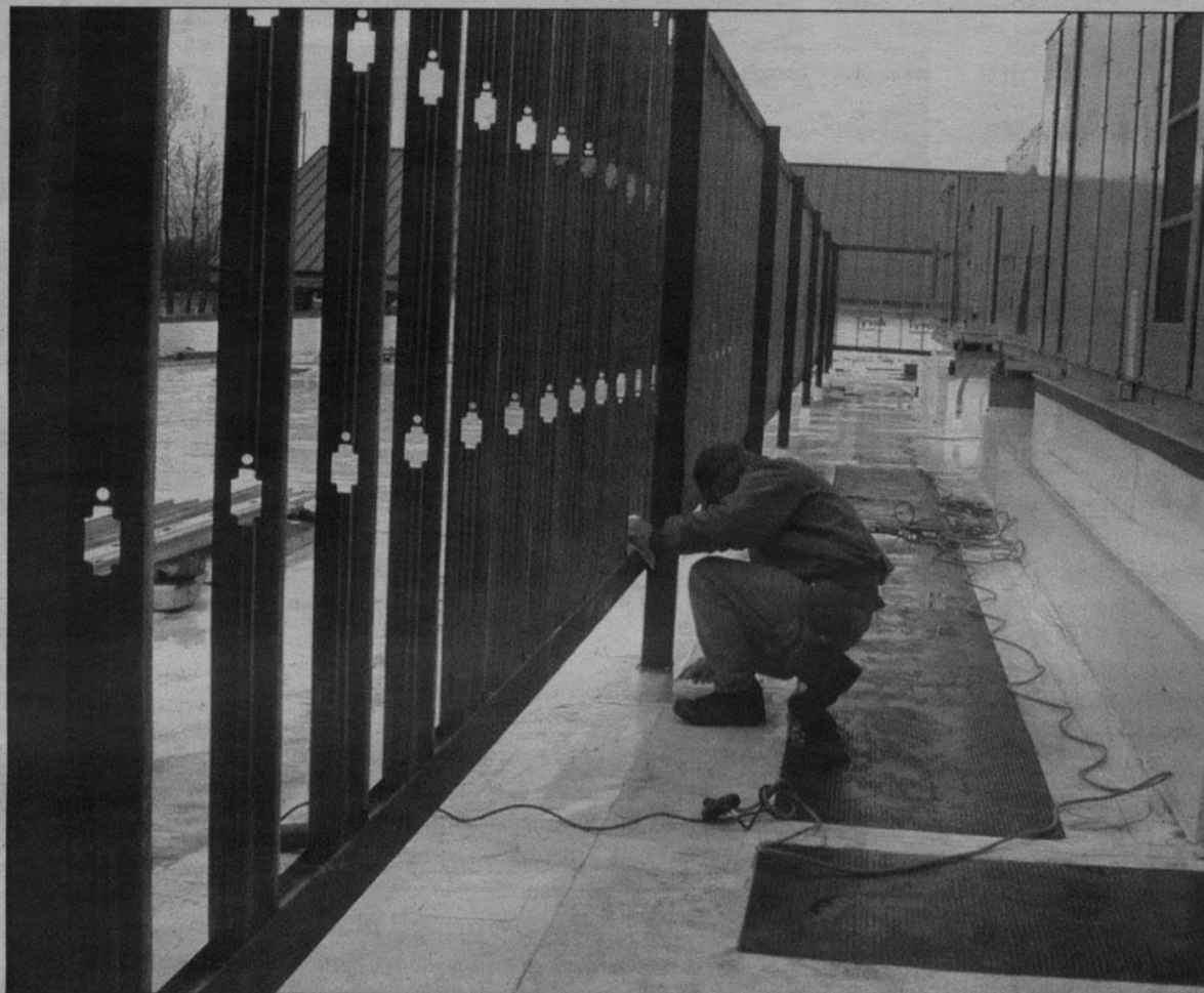
Workers install the heating and air-conditioning system on the roof of the new One Stop Center, which will become the new home of LBCC's Lebanon Center this spring.
