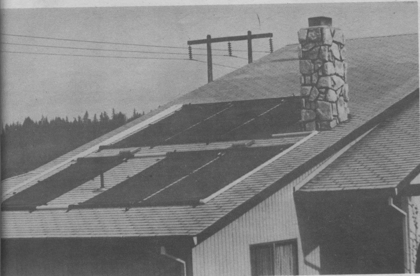
Solar panels on an Oregon rooftop are still a rare sight.
