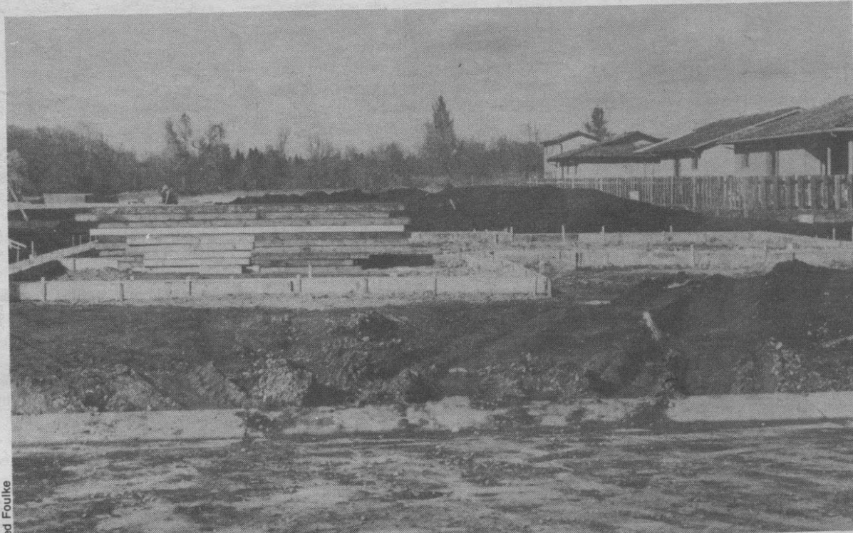
The construction technology class is in the process of laying a foundation for the house they are building just north of the campus.
