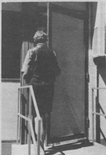
COMMUTER staff member Ellen Hillemann looks over damage caused to bookstore door by vandals.
