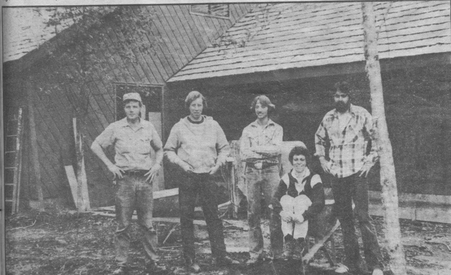
LBCC students show off the house they built. Student on the left is in refrigeration and air conditioning. Construction students are (continuing from left) Jim Gray, John Brumbaugh, Karen Marlin and Jim Bousquet. The 1,550 square foot, energy-efficient house at 1768 Belmont Loop S.W. will be for sale after it is appraised.
