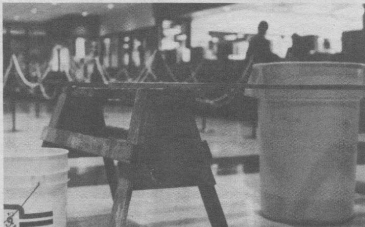
Barricades guard buckets catching leaks from the Tadena Hall roof.
